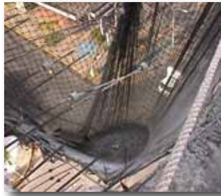
12 cubic feet of concrete caught by safety netting with debris liner.
